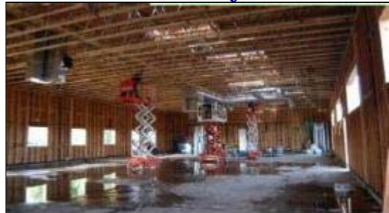
Construction on the Councilman Greig Smith LAPD Devonshire Area Youth Center in Northridge is well under way.
